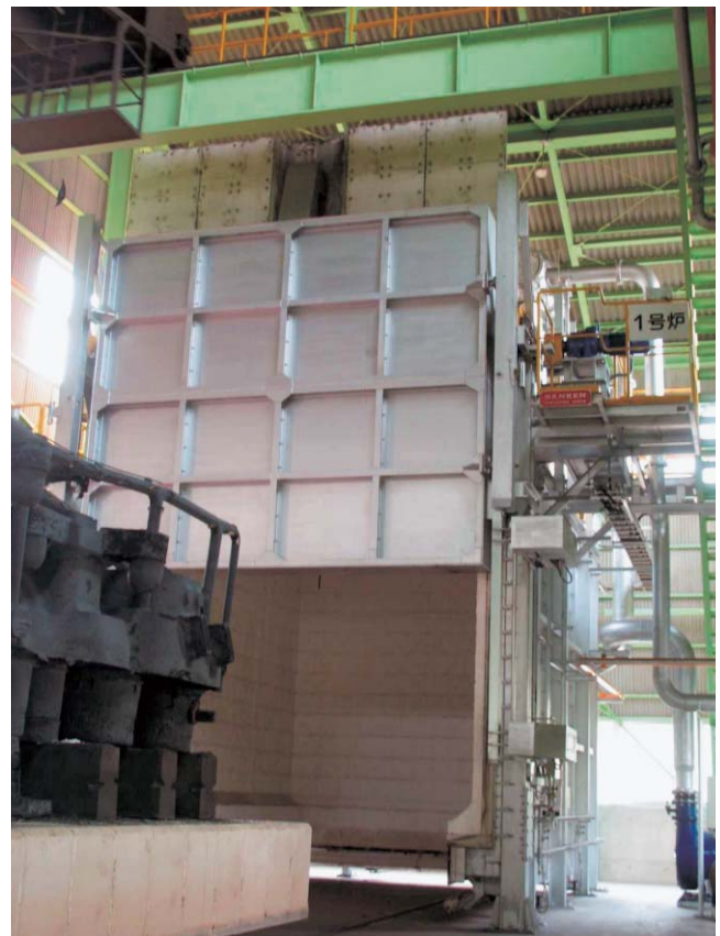
No.1 熱処理炉 (LNG専焼炉) No.1 Heat Treatment Furnace (LNG)
